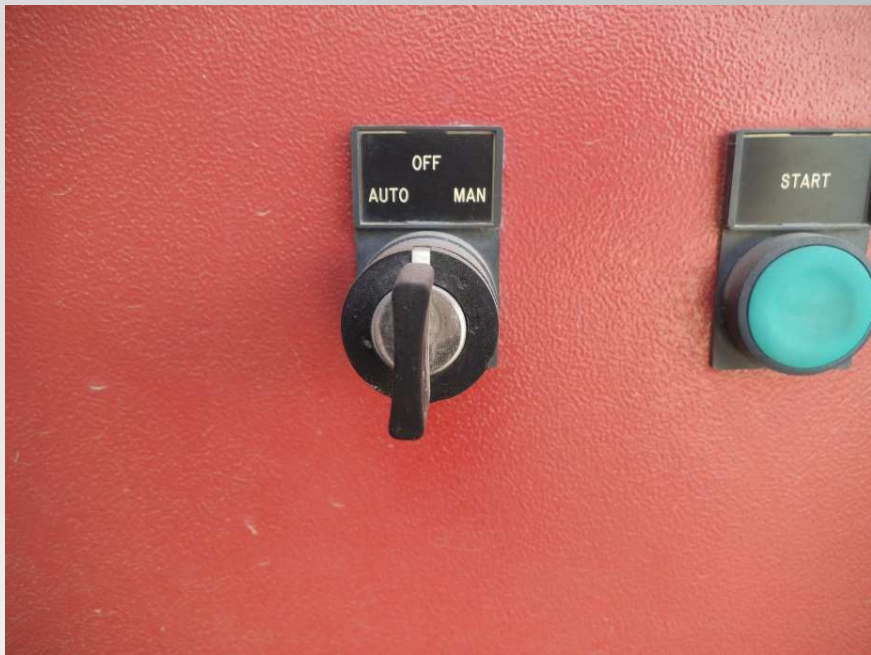
Fire Pump Controller Off
