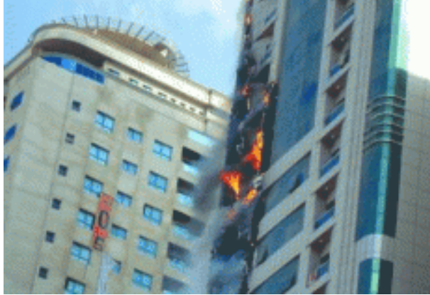
A fire gutted 17 floors of a 33-storey residential building in the Al Nahda area of Sharjah
